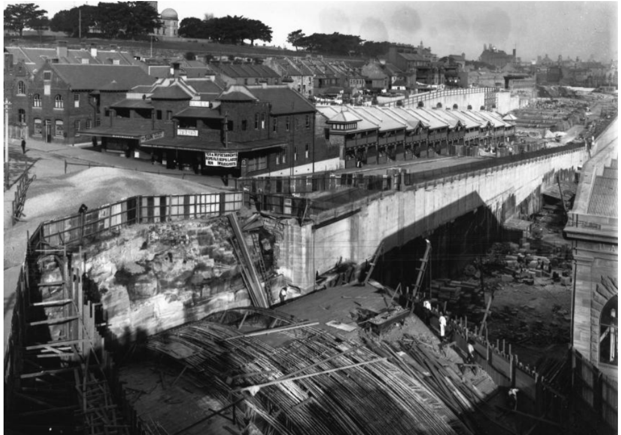
Construction of the Munn Street Bridge, Millers Point, 1912 [A-00014129]. Source: City of Sydney Archives
